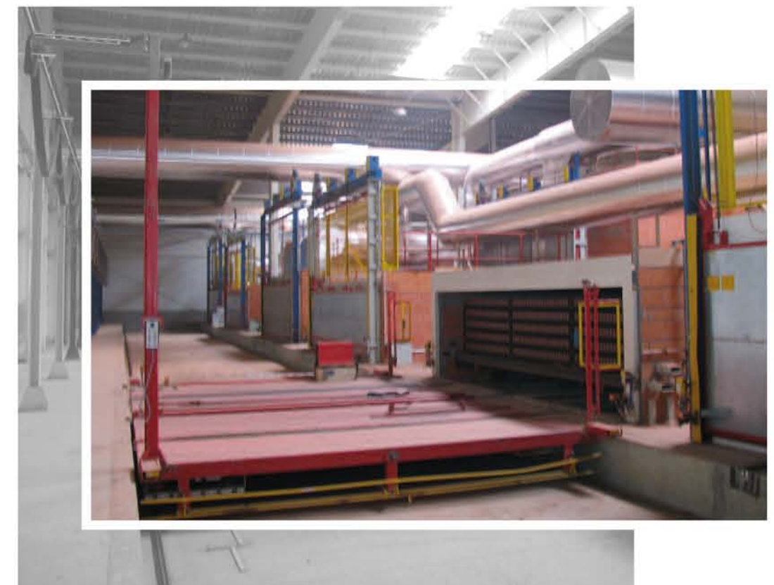
Dryer exit – kiln entry
