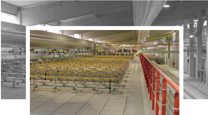
Top fired tunnel kiln
