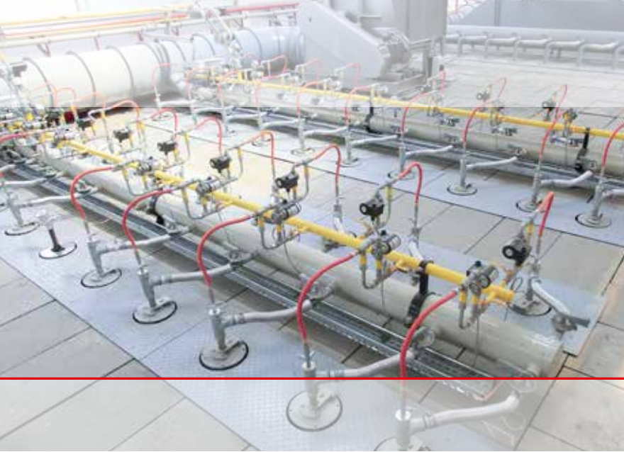
Burner groups for flashing
